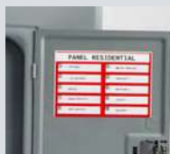
Residential panel labeling
