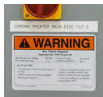
Arc Flash Panel Labels
