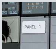
Control panel labels
