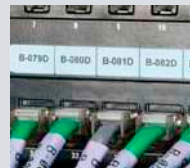
Patch panel and terminal block ID
