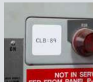
Asset and equipment ID
