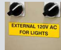
Equipment and panel labeling
