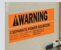
Equipment and panel labeling
